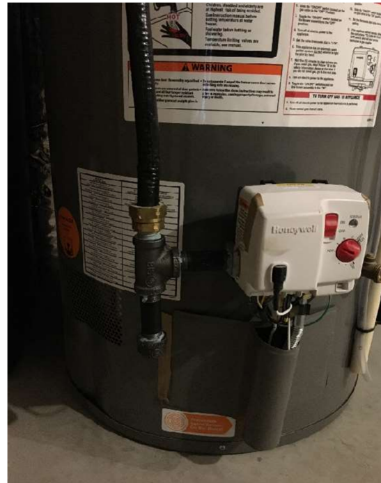
Water heater gas piping
