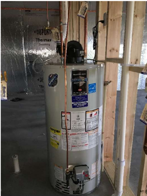
Water heater front view
