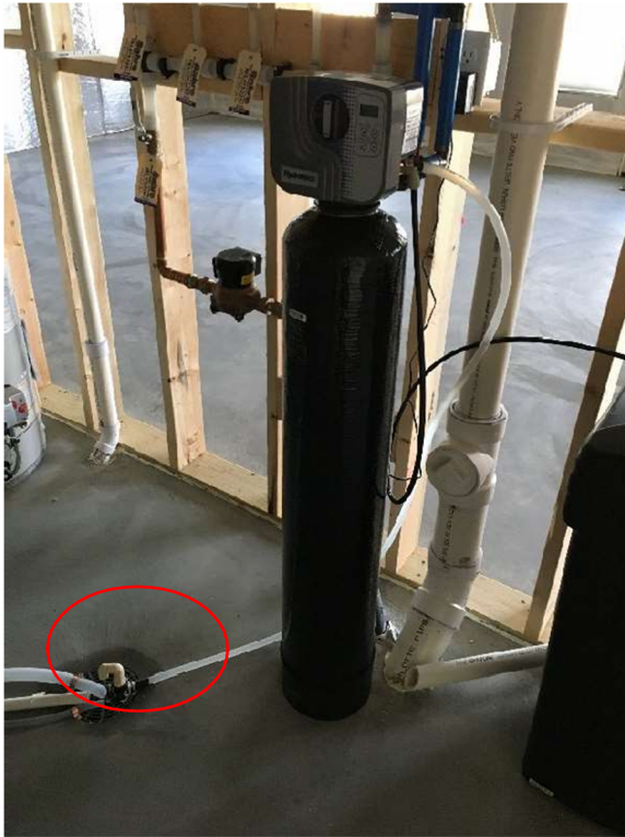
Softener front view
